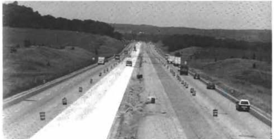
Traffic continued in 2 lanes while new 3rd lane and reconstructed dual lanes were done. Epoxy-coated rebar is in place on right inside lane.
