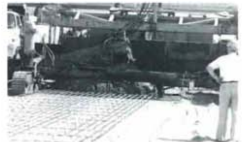
Spreading concrete over grade. Epoxy coated rebar was set on bar chairs for close placement control.
