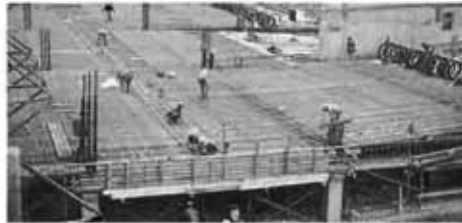
Installing epoxy-coated reinforcing steel on the third level. N. G. Jacobson & Associates specialize in the design of parking structures and specify epoxy-coated rebar for parking decks; even in warmer climates like Seattle where saltwater proximity could spell future problems.
