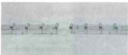
This shows the other method of placing epoxy-coated contraction joint assemblies on the road base ahead of the paving operation.
