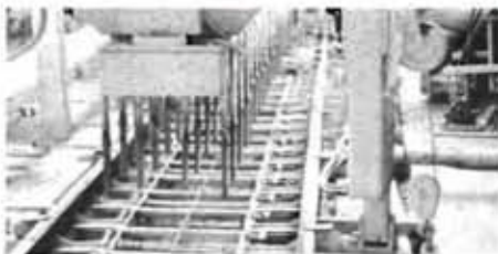
Mechanical insertion of epoxy-coated bars by the moving slipform paver is gaining rapid acceptance by engineers and contractors.
