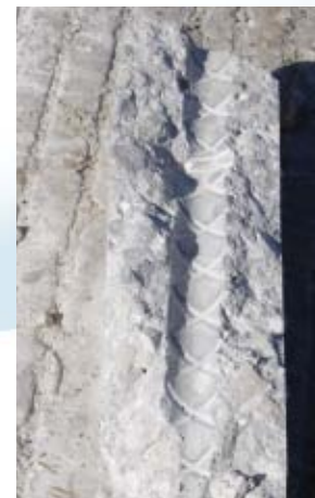
Concrete core sample with smooth, unstained rebar impression
